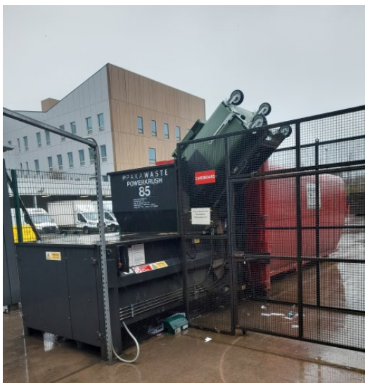
Photo 1: Compactor at DGRI loading waste from a wheelie bin
